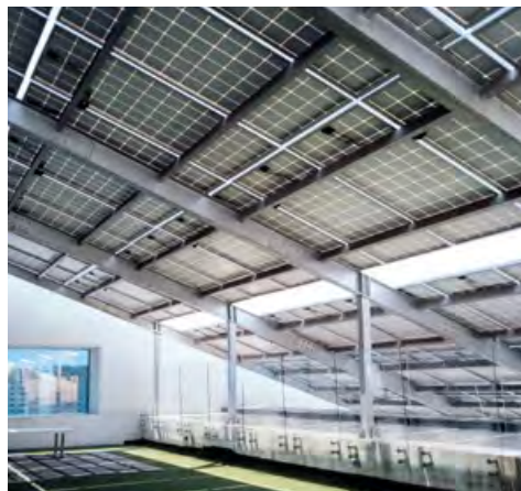
Solar panels on the roof of De Beers Group Industry Services Building, Surat.
