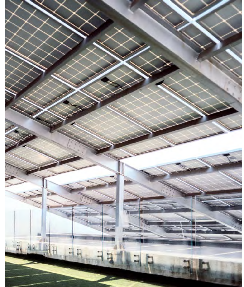
Solar panels on roof of De Beers Group Industry Services Building, Surat.
