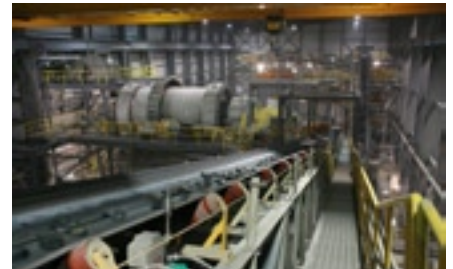
Conveyor and crusher in Snap Lake process plant
