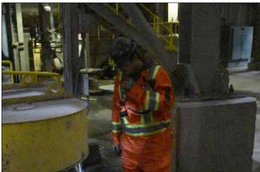
Morin Neyelle, a Process Plant trainee during 2024, inspects one of the pumps in the process plant.
